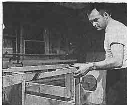
CHINE LOG JOINTS fall under joints in bottom planking and must be notched for 3/8-in. butt plates
