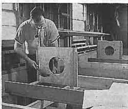
PLYWOOD BULKHEADS mounted on the 2 x 6 beams make up three building bulkheads spaced 4 ft. apart
